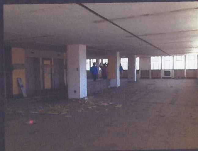
The space is cleared prior to the installation of the walling system
